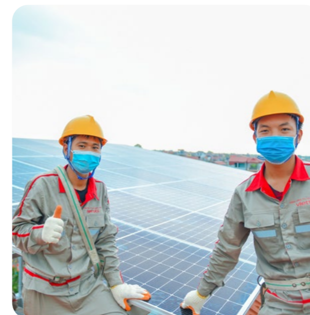
Operating solar system for VIETKING Import-Export Co., Ltd (1 MWP)
