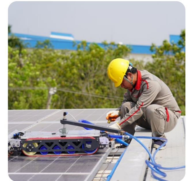
Cleaning and maintaining the solar energy system of V-KOM Quang Binh Investment Joint Stock Company (1 MWP)
