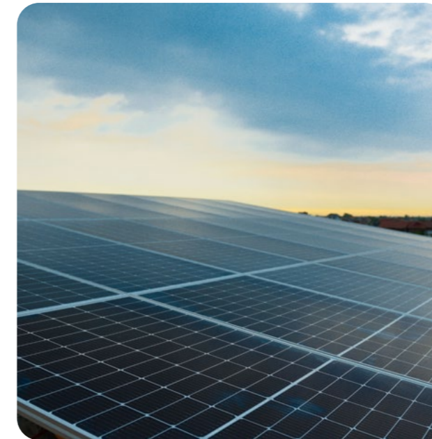
Operating rooftop solar power systems for CME Solar partners in 8 provinces (20.6 MWP)
